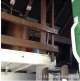
Unsafe Score Box Area
