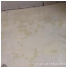
Damp on the external wall
